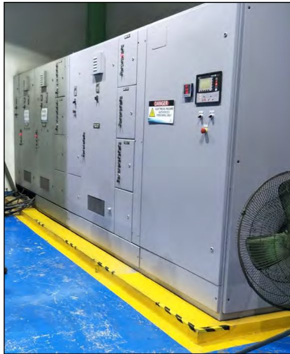
LV SOFT CLOSE TRANSITION ATS for MAYNILAD COMMONWEALTH BOOSTER PS
