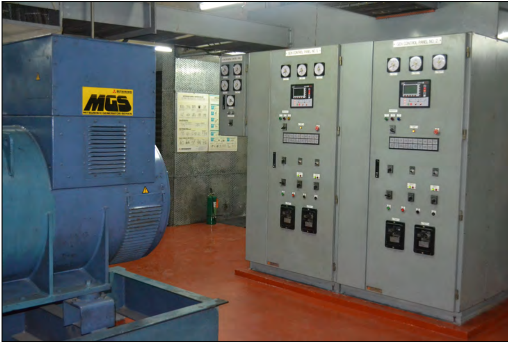
LV SYNCHRONIZING PANEL for NEW WORLD MANILA BAY HOTEL, MANILA CITY
