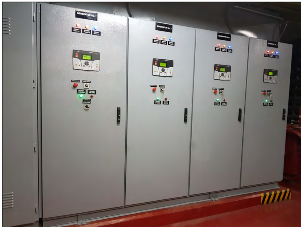
LV SYNCHRONIZING PANEL for INTERNATIONAL SCHOOL OF MANILA, BGC
