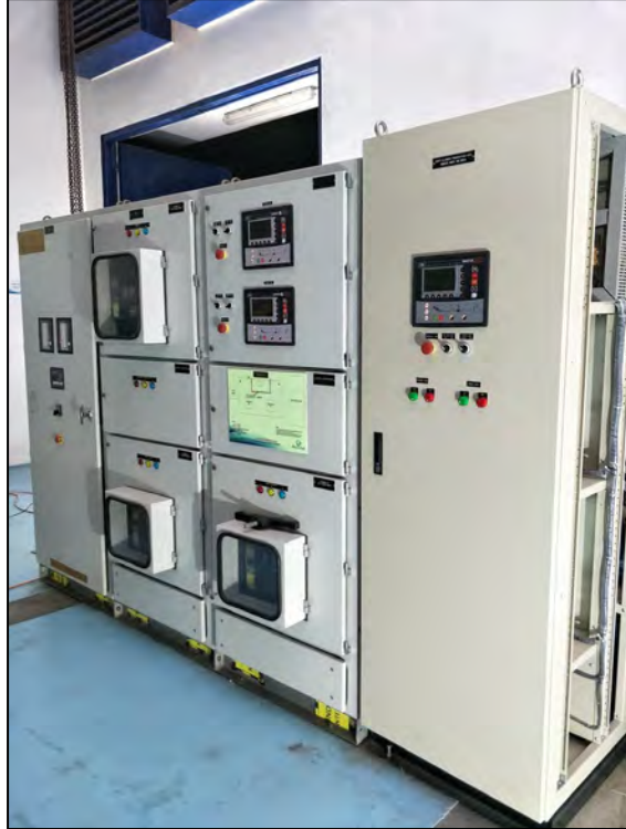
LV SOFT CLOSE TRANSITION ATS for MAYNILAD PATINDIG ARAW PS & RESERVOIR
