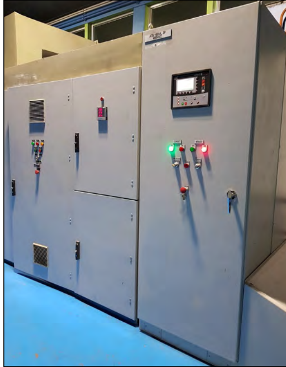
LV SOFT CLOSE TRANSITION ATS for MAYNILAD CALOOCAN PS & RESERVOIR
