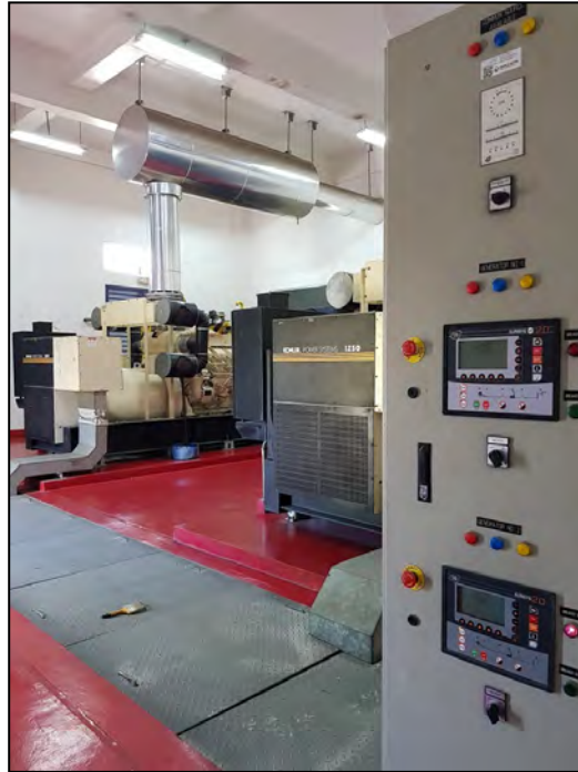
LV SYNCHRONIZING PANEL for MANILA WATER WTP, LITEX QUEZON CITY
