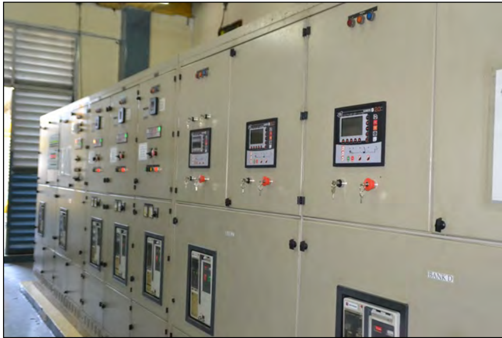
LV SYNCHRONIZING PANEL for ROBINSONS STARMILL, SAN FERNANDO CITY, PAMPANGA
