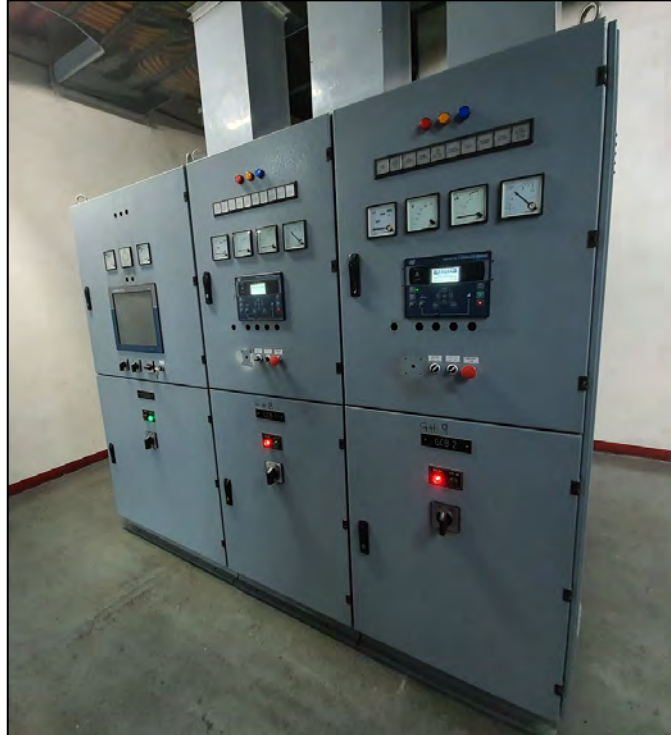
LV SYNCHRONIZING PANEL for SHANGRI-LA MALL, EDSA-SHAW, MANDALUYONG CITY
