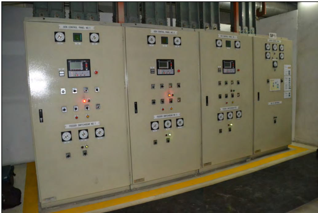
LV SYNCHRONIZING PANEL for THE ENTERPRISE CENTER TOWER 2, MAKATI CITY
