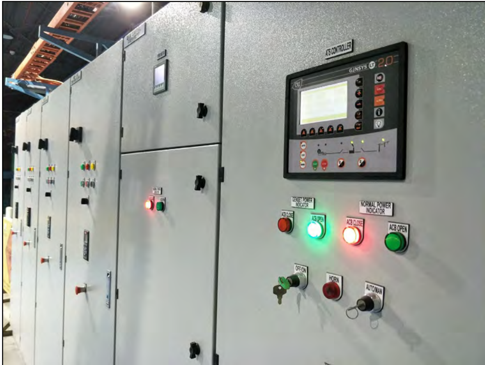
LV SOFT CLOSE TRANSITION ATS for MAYNILAD ERMITA PS & RESERVOIR
