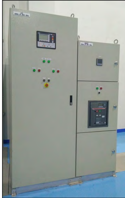
LV SOFT CLOSE TRANSITION ATS for MAYNILAD ALABANG ZAPOTE BOOSTER PS
