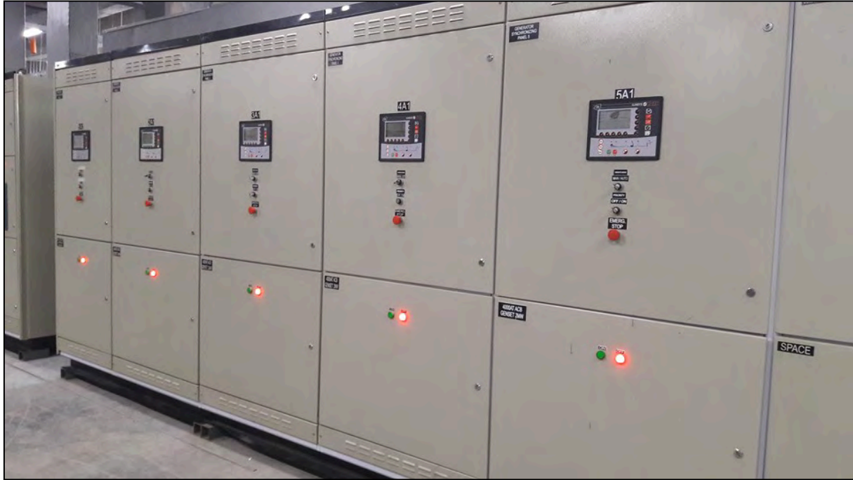
LV SYNCHRONIZING PANEL for KCC DE ZAMBOANGA MALL, ZAMBOANGA CITY
