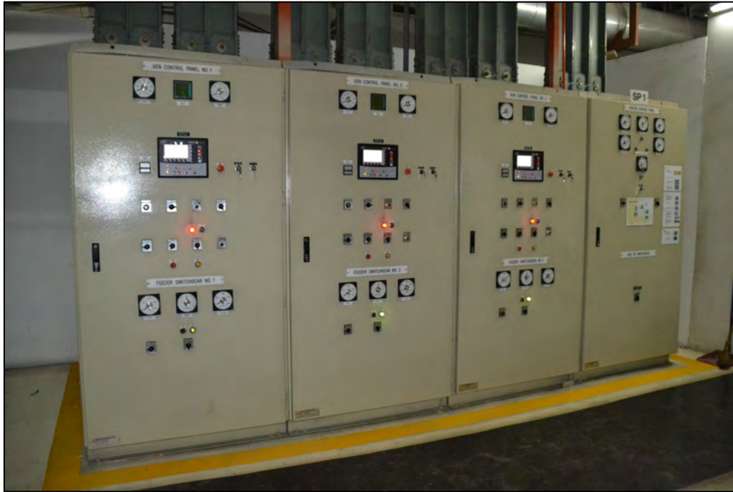
LV SYNCHRONIZING PANEL for THE ENTERPRISE CENTER TOWER 1, MAKATI CITY
