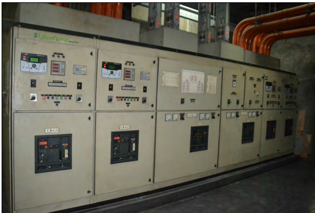
LV SYNCHRONIZING PANEL for ROBINSONS SUMMIT CONDOMINIUM, MAKATI CITY
