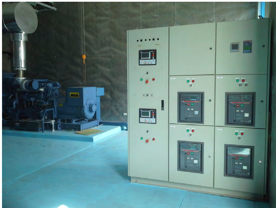
LV SOFT CLOSE TRANSITION ATS & SYNCHRONIZING PANEL for MAYNILAD MARCOS ALVAREZ BOOSTER PS
