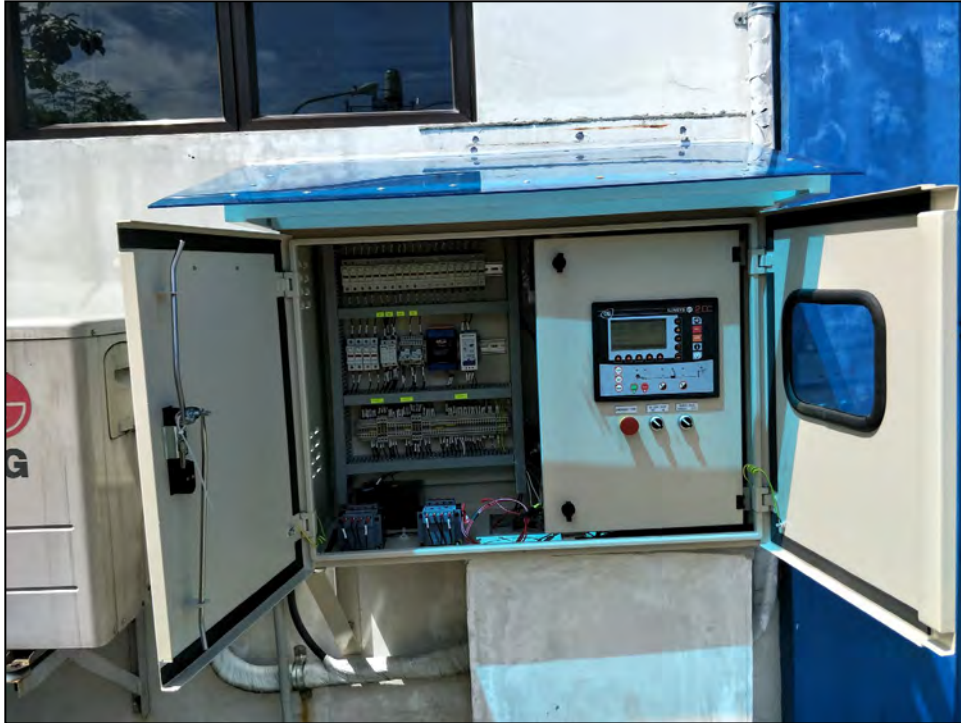
LV SOFT CLOSE TRANSITION ATS for MAYNILAD BAESA PS & RESERVOIR
