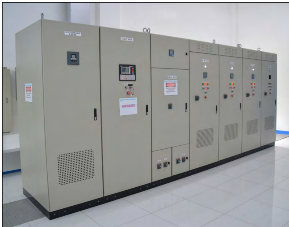
LV SOFT CLOSE TRANSITION ATS for MAYNILAD SACRED HEART PS & RESERVOIR
