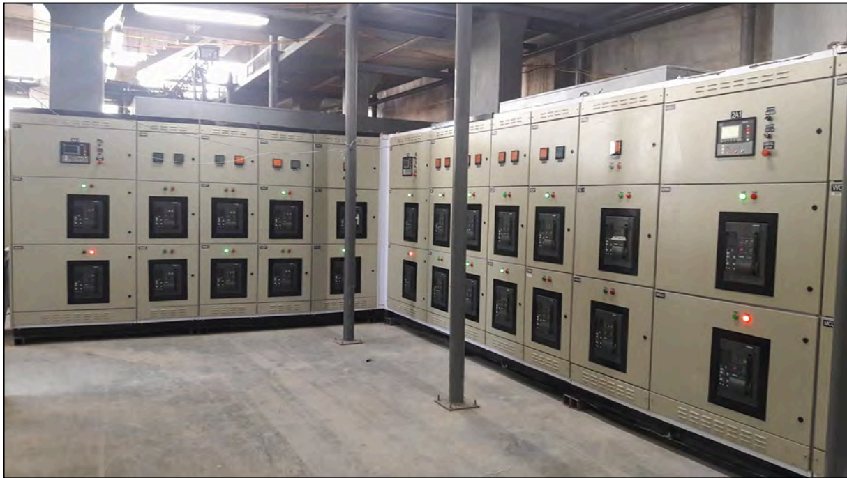
LV SOFT CLOSE TRANSITION ATS for KCC DE ZAMBOANGA MALL, ZAMBOANGA CITY
