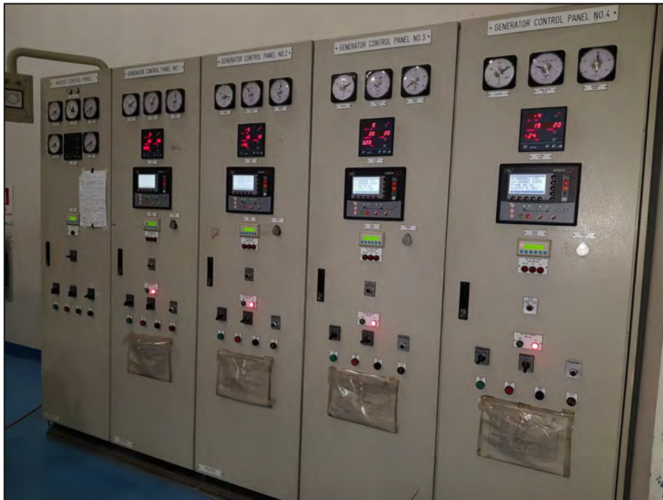
MV SYNCHRONIZING PANEL for LAMESA NORTH A, B, C BOOSTER PS
